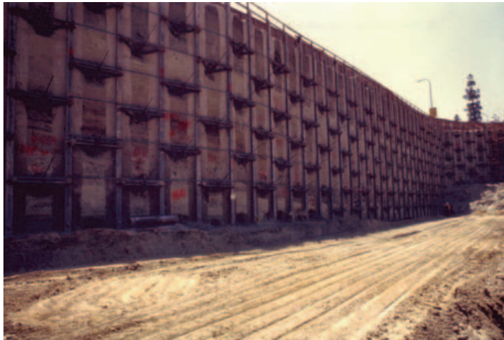
Figure 4. Tie-back Anchor Shoring System for Century City Theme Towers; note that the excavation was still not at full depth (circa 1970)
